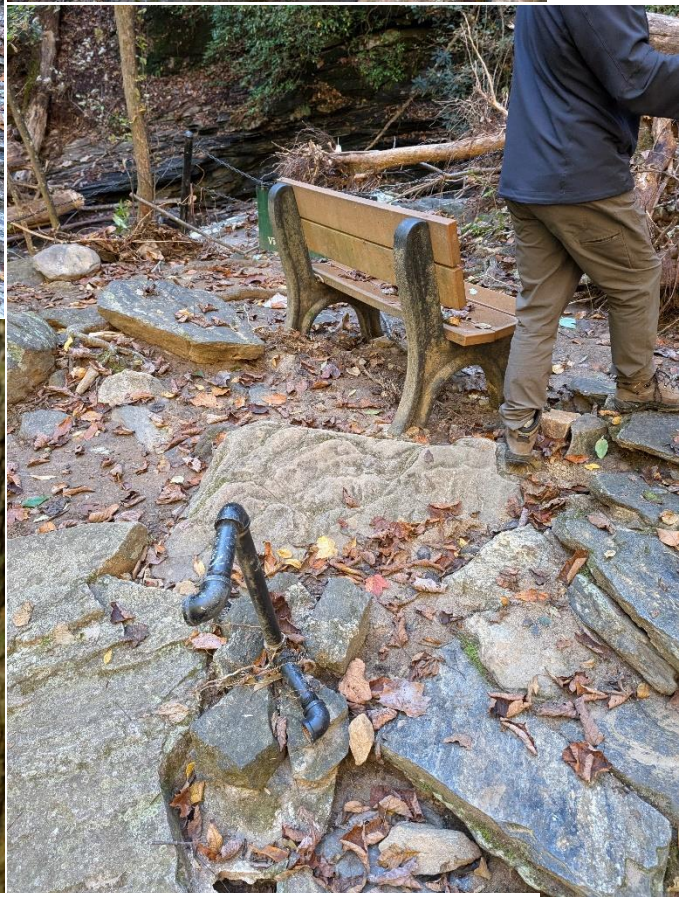
Top L: Debris under Chase Bridge. Top R: The landslide with a red arrow indicating a person. Bottom L: Debris where the trail once was. Bottom R: Susan Kelley's bench at the falls and what is left of the railing.
